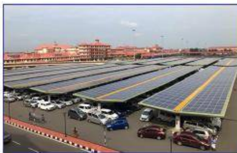
The Solar Power Plant at the International Airport, Nedumbassery. The Power Plant takes care of the complete energy needs of the airport and the excess energy is given to KSEB. It received the Champion of Earth Prize – 2018 instituted by the United Nations for its use of Green Energy.
